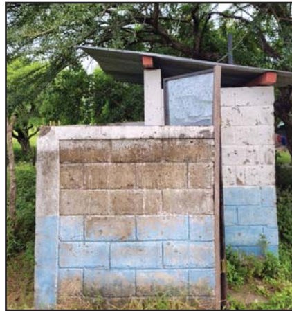
Non-working latrine to be replaced.
