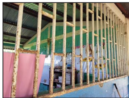
Screening will cover these windows and keep out trash, leaves and bugs.
