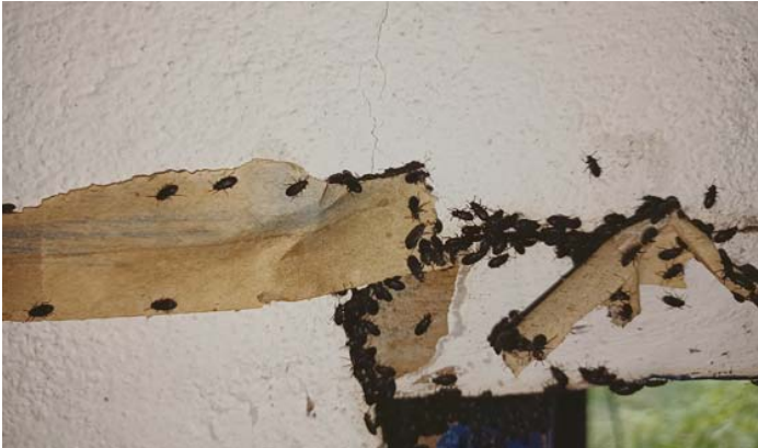
Some of the damage from insects that have infested the ceiling panels and wood structures at the primary school in El Platanal.
