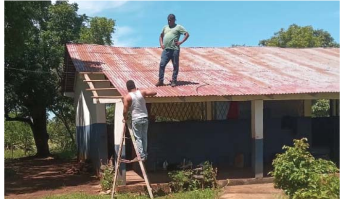
Work to renovate and improve the building that houses grade 5 and the pre-school kids started on September 26, 2023.
